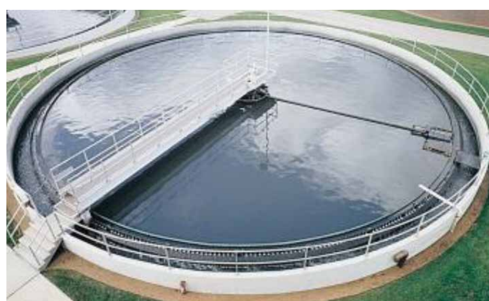
Water Treatment Tanks
