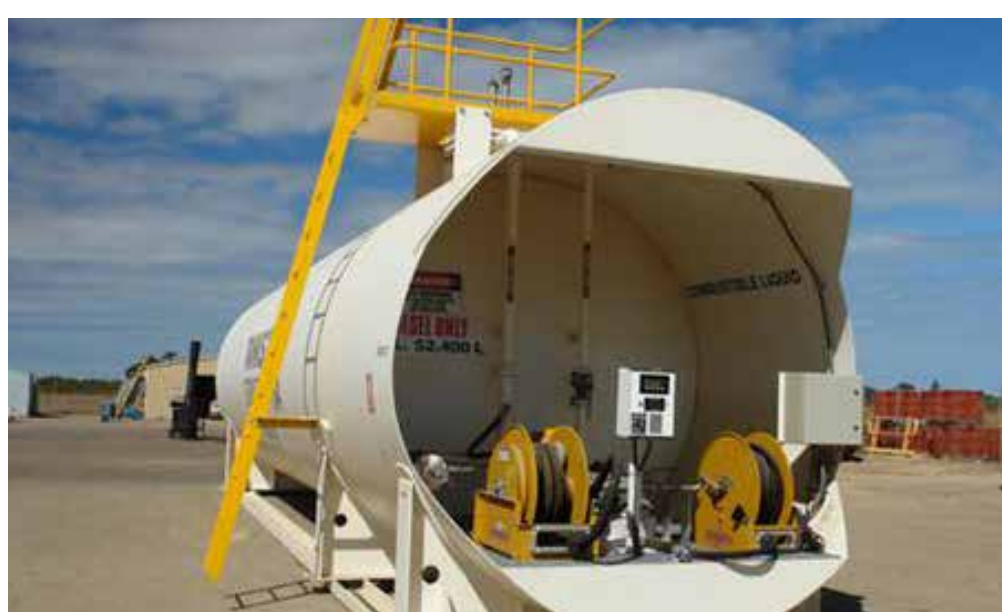
Bunded Fuel Store and Fill Station
