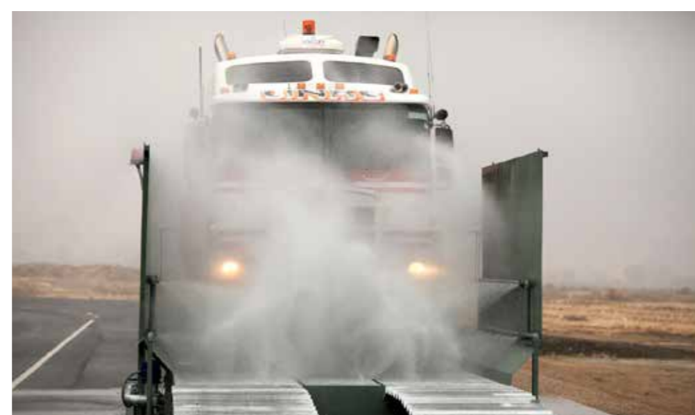
Truck wheel wash bay
