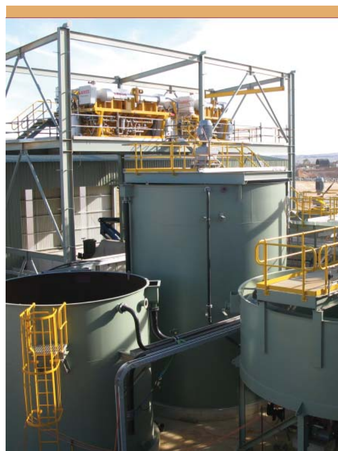
The Angas process plant - concentrate thickening and filtration section.
